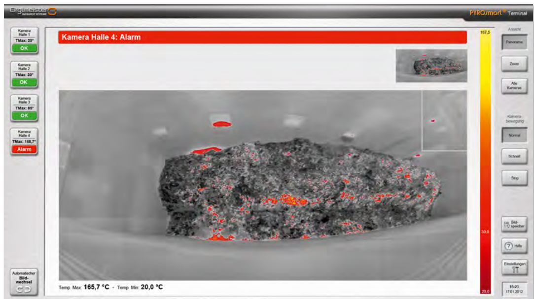
IR panorama image of a waste bunker and touch-screen operating panel
