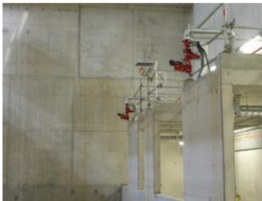
Image (Löschwerfer.jpg): PYROsmart detects critical temperatures in the waste bunker and, in the event of a fire hazard, controls the automatic deployment of extinguishers.
