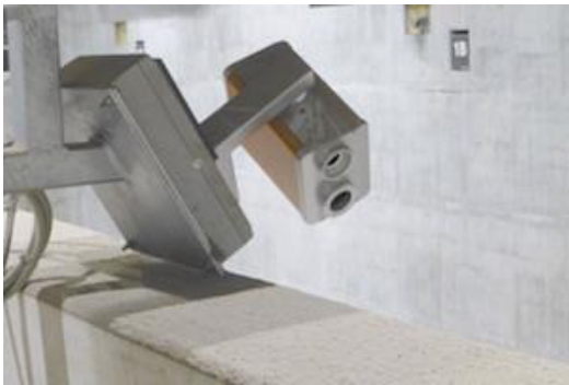
Image (Müllbunker.jpg): PYROsmart unit during the scanning process for fully comprehensive monitoring of a waste bunker.
